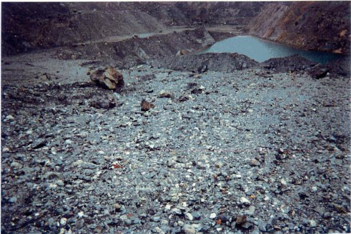
PLATE 4. SLIDE DEBRIS ON ROAD DOWN TO SOUTH PIT (NORTH), SHOWING ENTRY POINT
